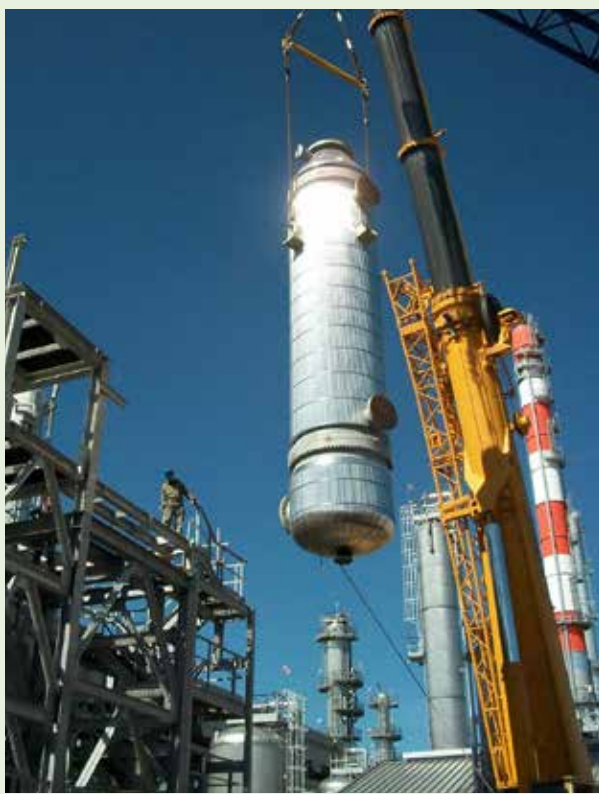
New depropanizer reboiler
